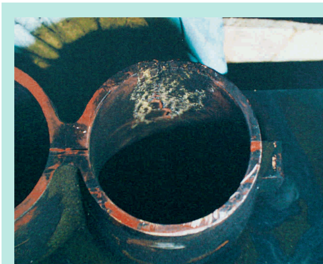
Failed 11kV Spout
