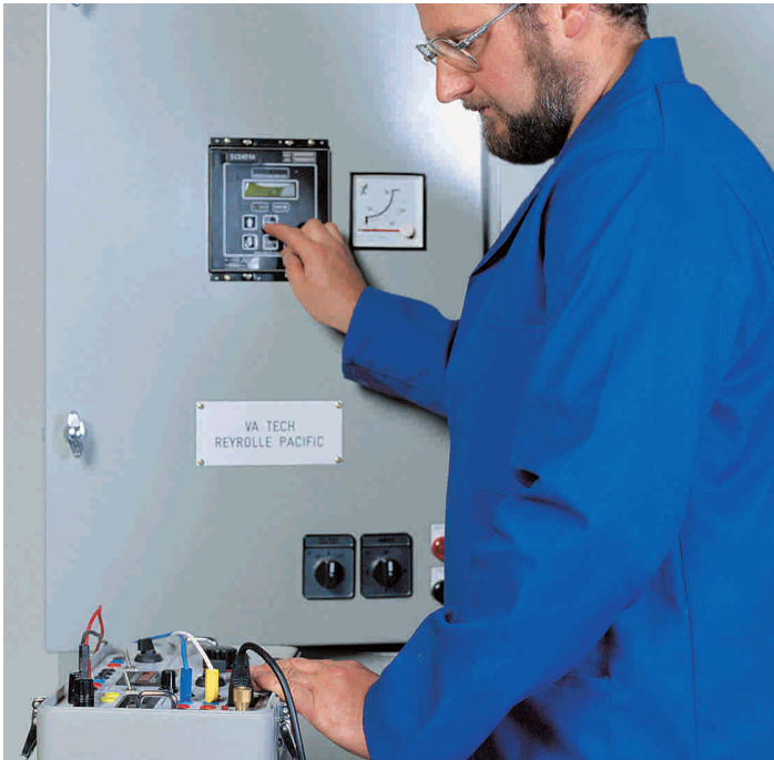
Commissioning tests on protection relay fitted to LMVP switchboard.
