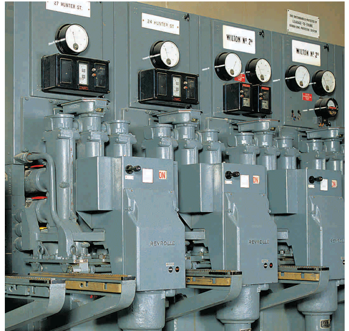
Reyrolle Type C gear still in service. This range of switchgear was manufactured from 1906 to 1970.
