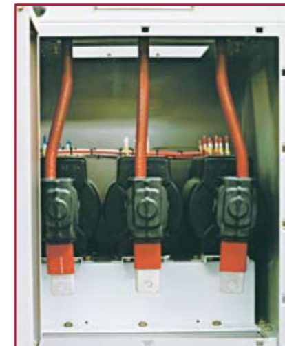
Single cable box with circuit connected voltage transformer housing fitted. (Covers removed to show internal details.)
