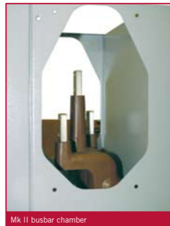
Mk II busbar chamber
