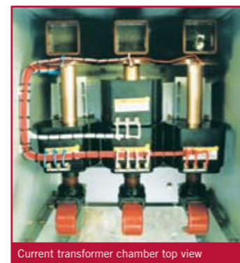
Current transformer chamber top view
