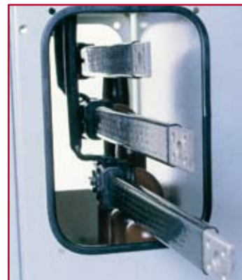
Mk 1 Busbar chamber with interconnecting busbars and associated busbar shrouds in position. Busbar connected VT risers can also be seen.
