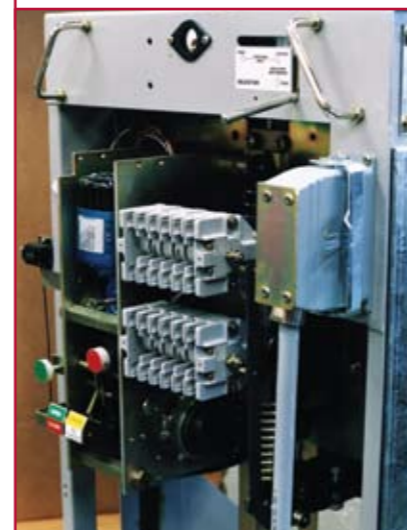
Motor charged spring mechanism – cover removed. (Type QMRO, RPM series circuit-breaker.)
