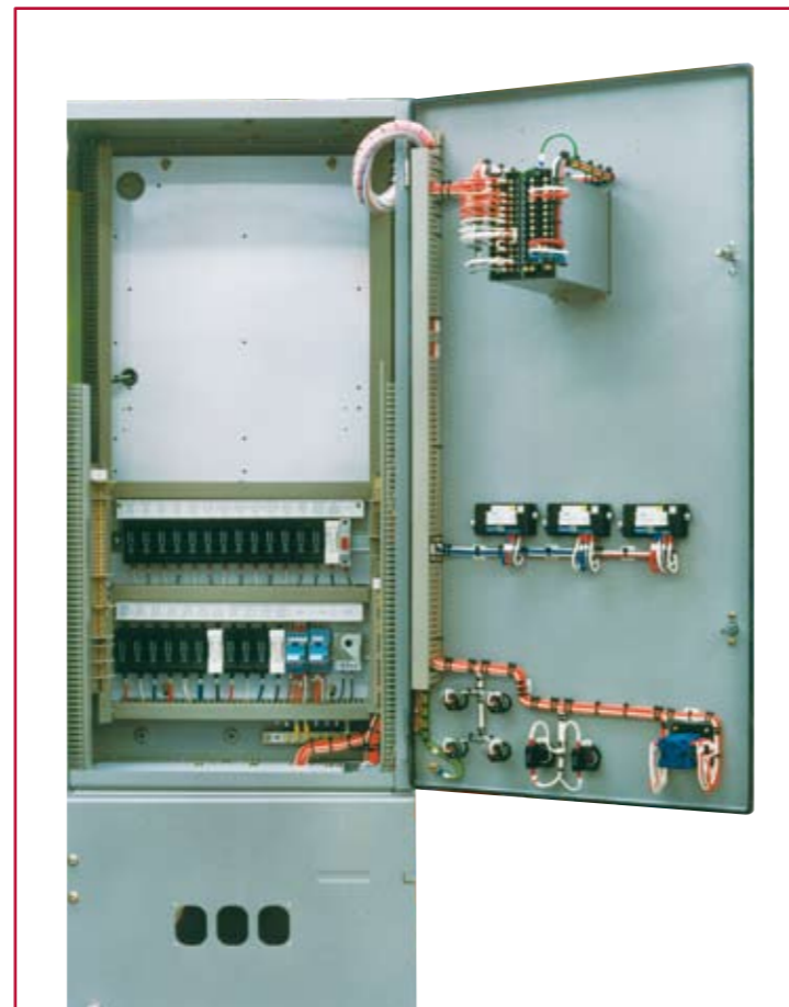
Photo of interior view of control section
